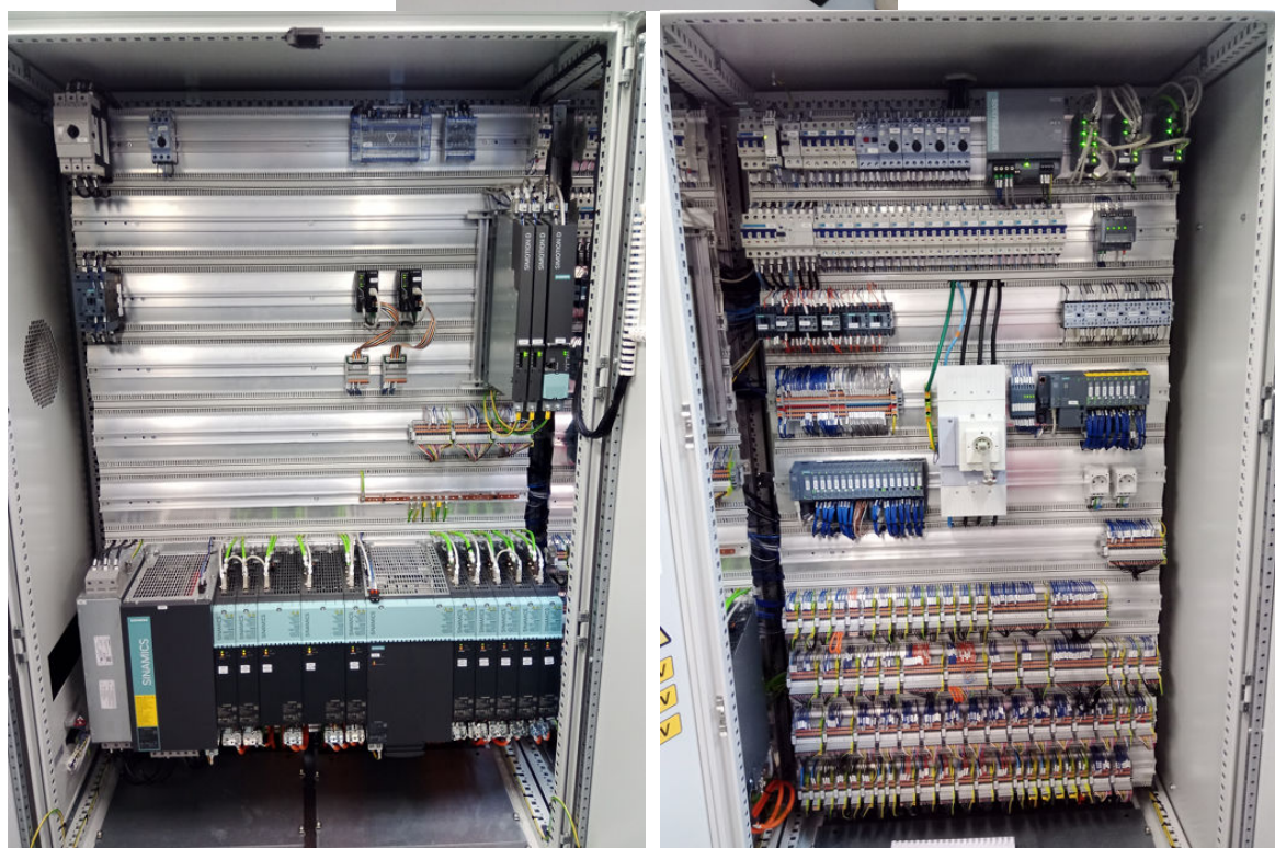
Painel Elétrico Principal
